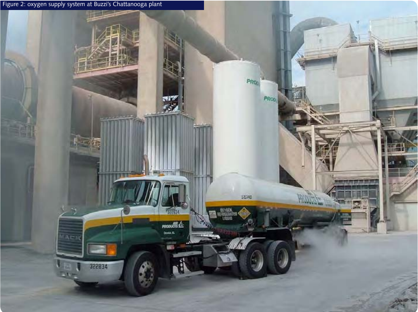
Figure 2: oxygen supply system at Buzzi's Chattanooga plant
