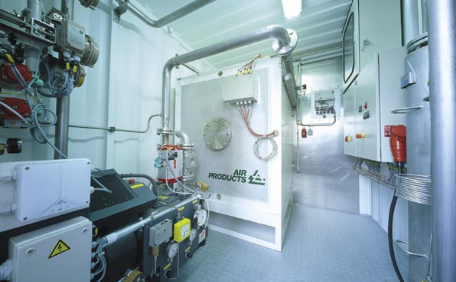
Main components of the “off-line” fluorination system
